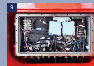
Electrical control system
